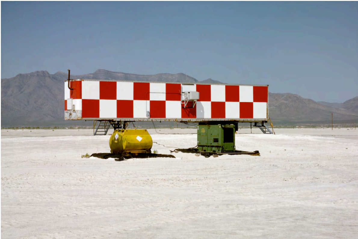
Figure 4. View of Xenon Control Trailer, Runway 17/35, looking west towards San Andres Mountains, showing detached generator and transformer, July 2003 (Source: NASA WSTF).
