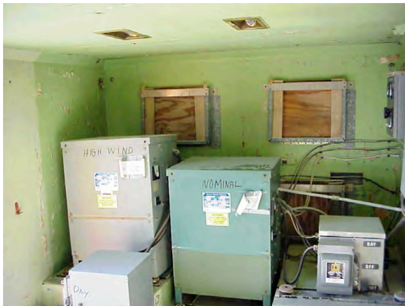
Figure 4B. View of the interior of the original PAPI Control Building, undated (Source: NASA WSTF).
