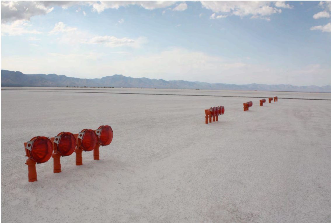
Figure 15A. View of Inner Glide Slope (IGS) Indicator Ball/Bar Lights on Runway 17/35, looking West towards San Andres Mountain Range, 2011.
