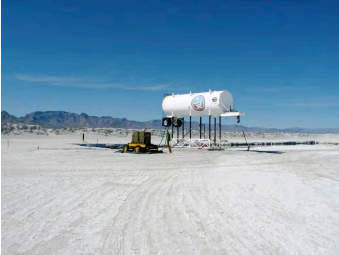
Figure 5. View of mechanical pumping equipment and portable generator at the Waterhole, looking northwest towards San Andres Mountains, February 2006 (Source: NASA WSTF).
